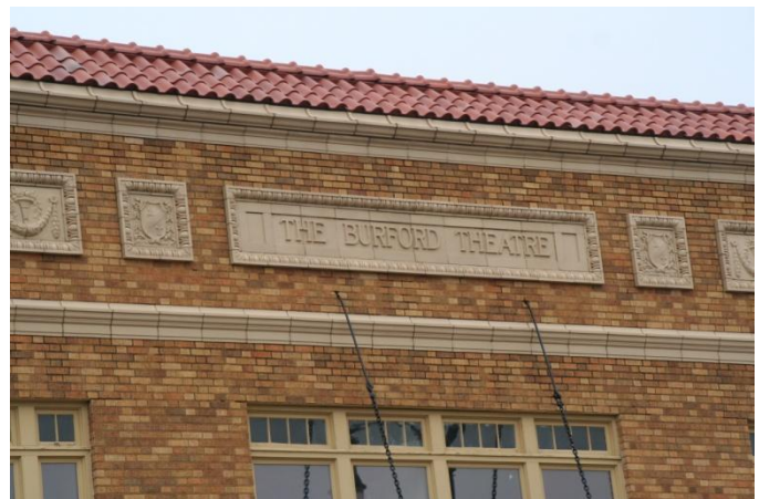
The Burford Theater and office building are among the few historic buildings in the district that have taken advantage of available preservation-based financial incentive programs.
