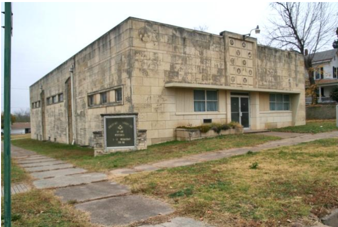
Built in 1954, the Masonic Lodge on E. 5 th Avenue is an excellent example of Post-WWII Era Modern building featuring subtle detailing with contrasting stone panels and horizontal bands of windows.
